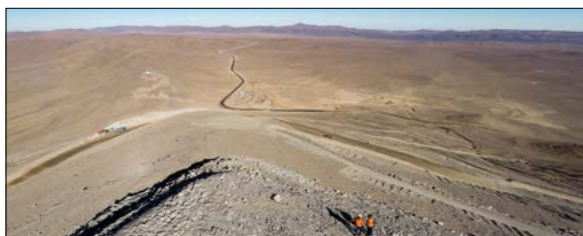
Drone-shot over Cerro Armazones, 3060 m altitude and 20 km from Paranal, the site where the construction of the European Extremely Large Telescope has started. The Argentinian Cordillera with the Llullaillaco volcano are visible in the background.
