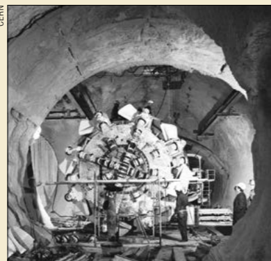
The mole being installed underground at the point where boring is beginning. Its 7 km journey around the ring is expected to be completed by autumn 1974. The machine, 80 m in length, comprises the 4.8 m diameter head, shown here, pressure and supporting pads, an operator's cabin, electrical equipment, conveyor belts, tunnel-lining system, skip changer and spoil-removal train.
